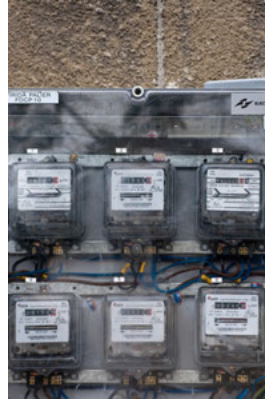
Figure 4.3: Electricity meters outside a building
